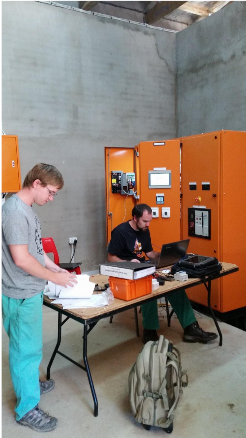
Control Panel being commissioned
