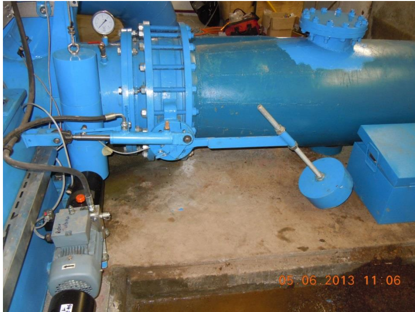
500NB Butterfly Main Isolation Valve
