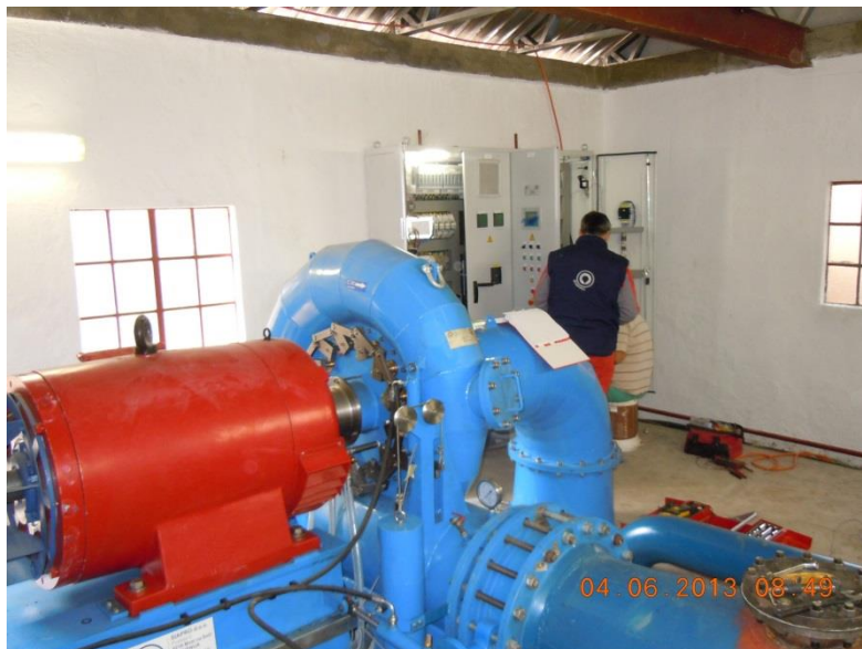
Turbine generator during cold commissioning
