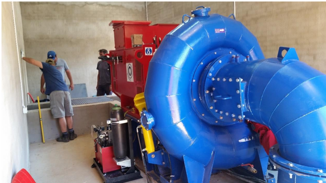
500kW Turbine Generator
